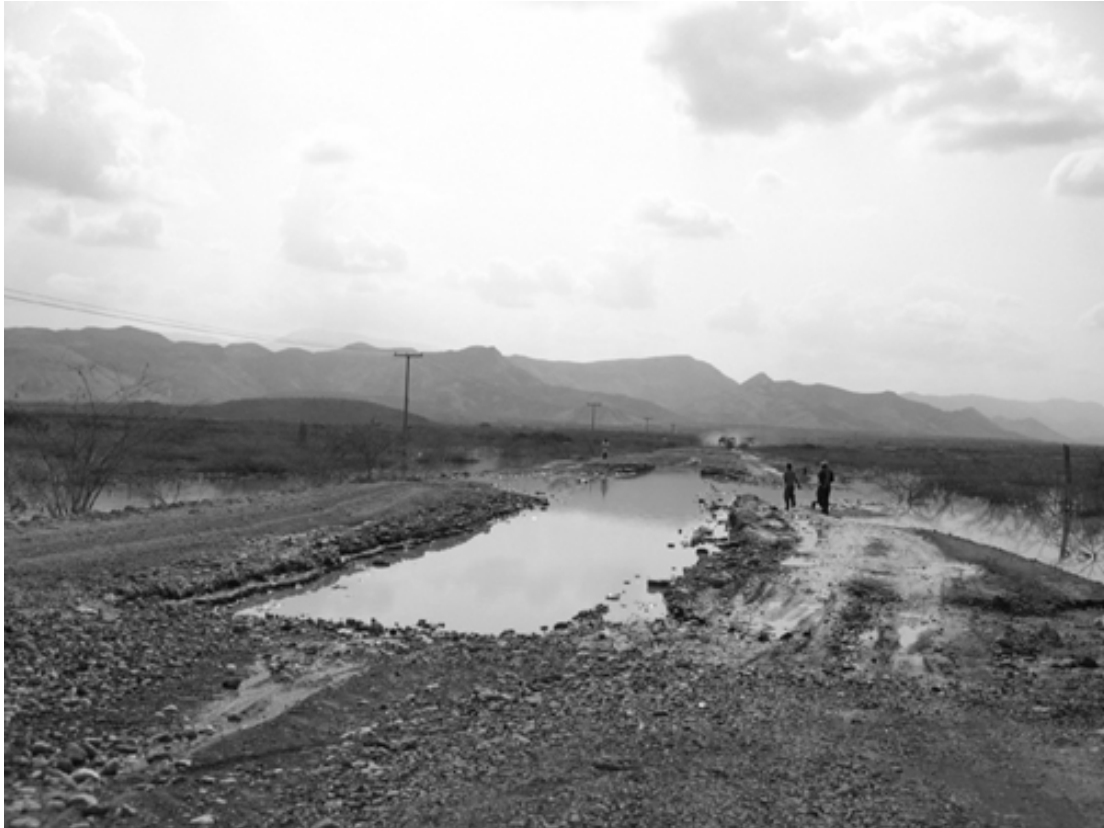
Damage to National Route #1, nine months after Tropical Storm Jeanne
